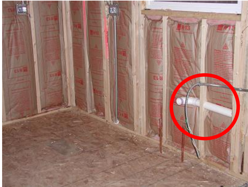
Figure 1.1.5 – Misalignment of insulation due to compression
