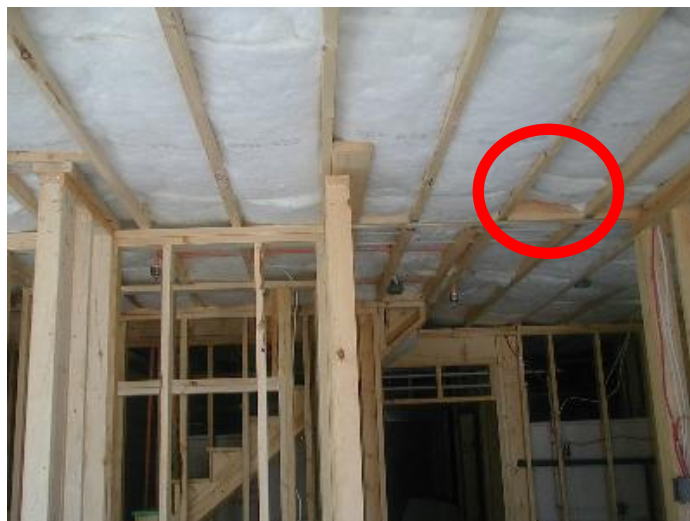
Figure 1.1.6 - Insulation installed with gaps and voids
