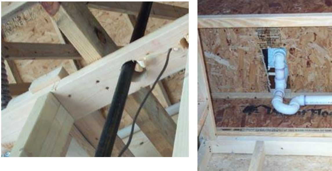
Figure 4.2.1 – Typical piping penetrations leaving large holes
