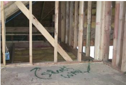
Figure 2.4.4 – Attic knee wall with no exterior air barrier
