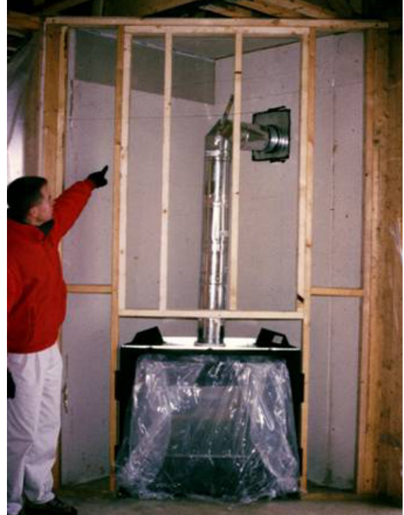
Image courtesy of Building Science Corp
