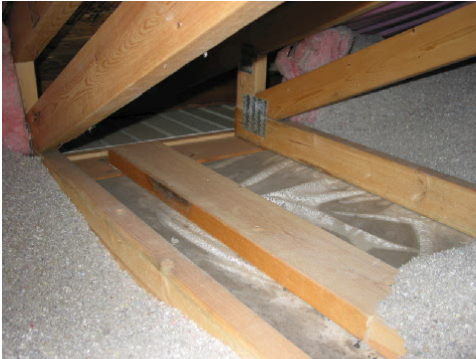
Figure 1.3.1 - Wind intrusion from a soffit vent
