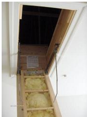
Figure 5.2.2 - Improperly installed insulation is compressed and impedes the use of the drop-down attic access stair.
