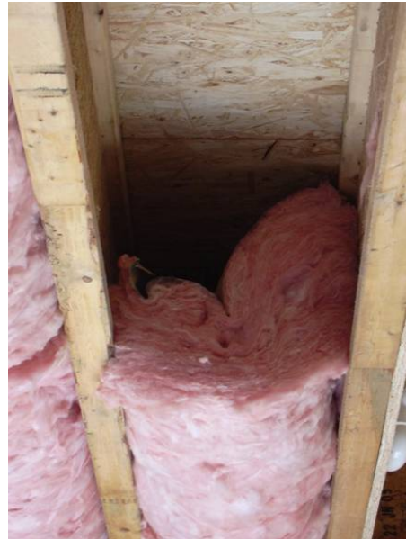
Figure 3.2.2 – Insulation settling away from sub-floor
