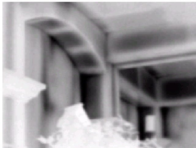
Figure 5.3.2 – Infrared image of dropped ceiling without an air barrier and proper insulation
